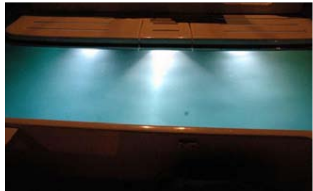
Image shows three lights, the one in the center does not have a diffuser.
